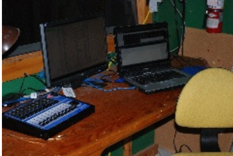
Lighting controls at Lighting Operator's Work Station. The Entec Playback wing is the console on the left.
